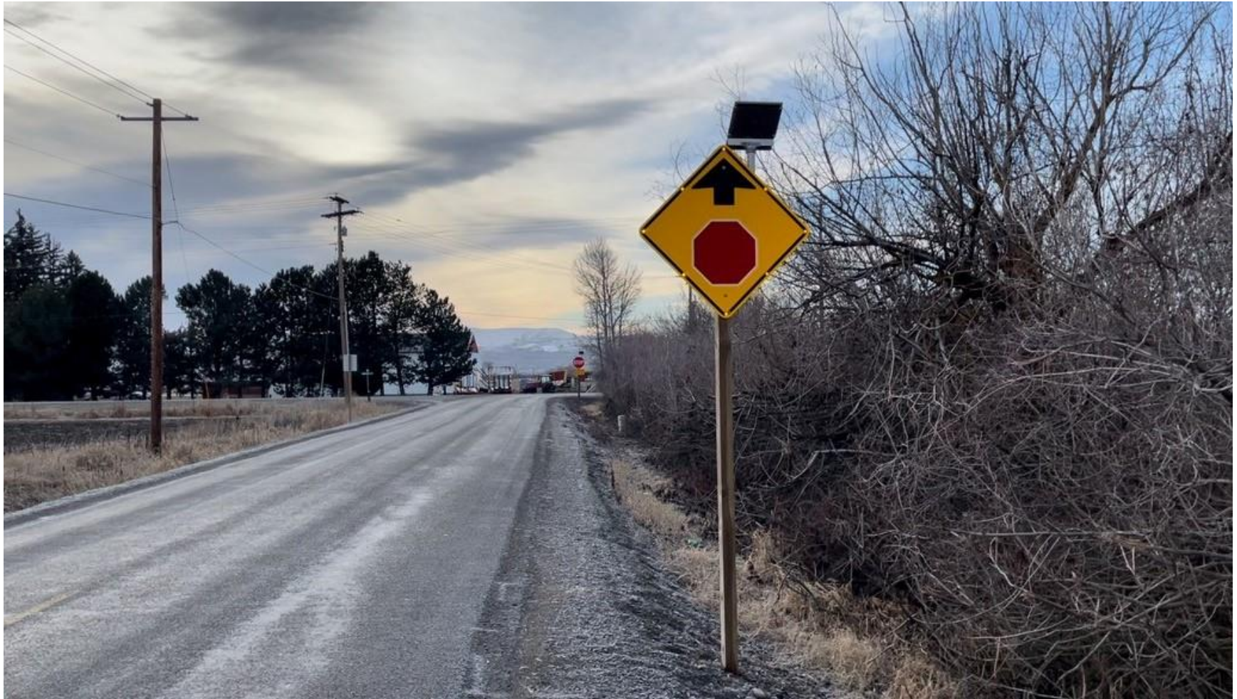
Naneum Rd LED Stop Sign Warning
